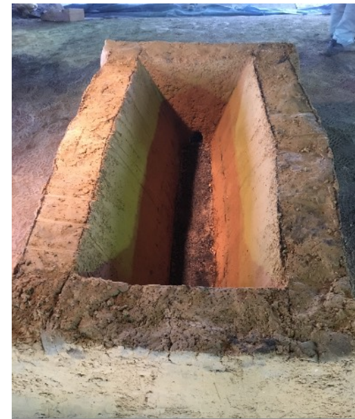
The lower section of the Niimi furnace was made wider before the side walls were built up to around 1.2m high.
